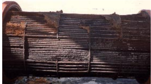
Fouling reduces heat transfer and increases pressure loss
